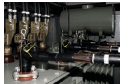
Transformer connection with 158LR
