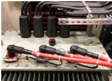
Transformer connection with 200LR
