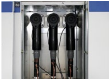
SF-6 system connection with 480TB
