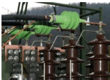
AFN10 as a transformer connection
